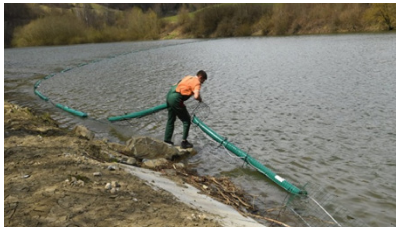
Figure 3. Installation of floating trash barriers in the area of the Ružín water reservoir
